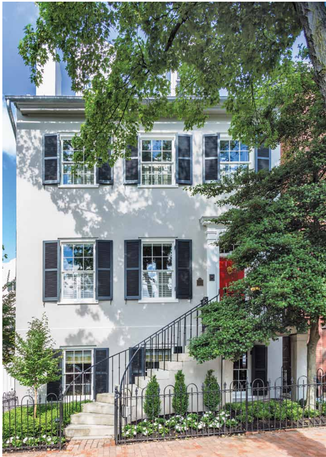
Barnes Vanze Architects meticulously restored the windows and façade to their original Georgetown elegance, capturing the bowing bricks by building an interior-reinforced concrete shell.
